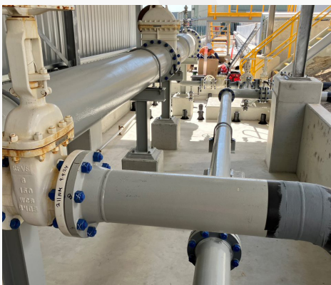
Hazardous banded area cluttered with exposed pipes and valves
