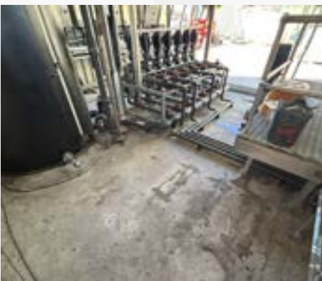
Safety Concerns | Limited Access
